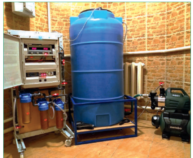
Fig. 6.2.9. EMERALD-UNIVERSAL-500 device as the main universal system for water purification and conditioning in a cottage. When the sensor of the lower level of purified water in the storage tank is triggered, water from the well with a constant flow rate of 500 liters per hour enters the storage tank, having previously passed all the stages of purification in the EMERALD-UNIVERSAL-500 device. When the upper level in the storage tank is reached, the EMERALD-UNIVERSAL device turns off. A pressure boosting station connected to a storage tank and connected to an in-house water distribution system provides the entire cottage with clean water at any time and in any required amount.
