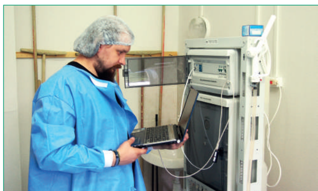
Fig. 6.4.2. STEL-ANK-SUPER-100 devices with Anolyte ANK SUPER capacity of 100 l/h, with automatic systems for maintaining the Anolyte level in the storage tank and cleaning the reactor. City Clinical Hospital No. 52, 2016
